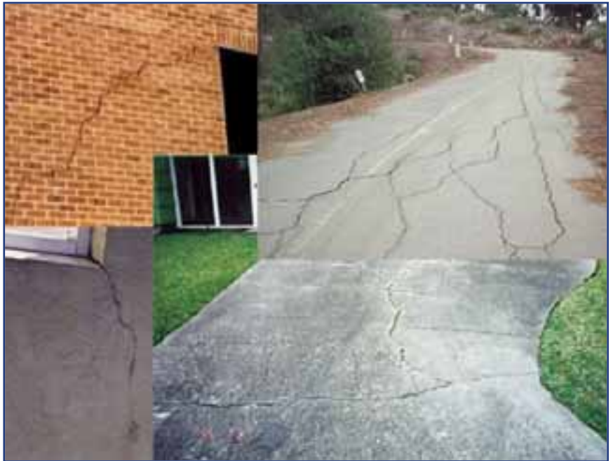
Figure 1: Damage induced due to shrink-swell in unsaturated soils
