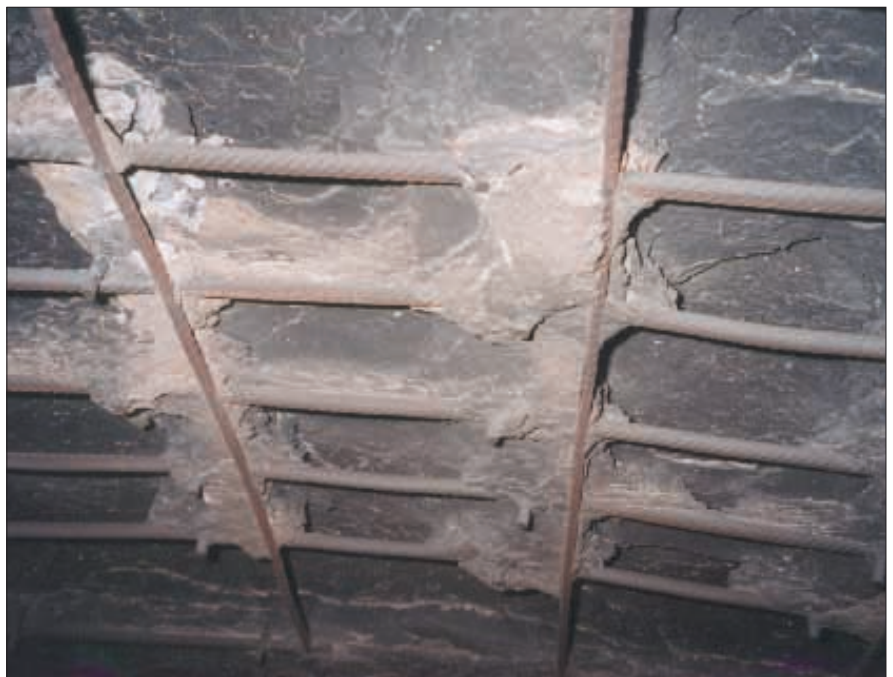
Figure 2: Spalling in the vault of the tunnel
